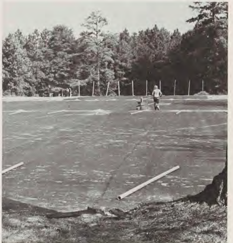
Outdoor sports have also received new facilities. Eight tennis courts were finished this fall, taking the place of the four courts facing east-west on the Richmond side of the campus. The new courts face north-south, and alleviate the problem of sun in the eyes. Construction on a $175,000 all-weather Chevron track having eight, 48-inch lanes was also begun this fall.
