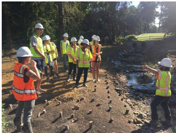
Image 3: University of Richmond students collect data in Little Westham Creek pre-restoration (above left, 2017, photo courtesy of RES). The location of Little Westham Creek on University of Richmond property provides opportunities for student and faculty research and community-based learning through invasive species removal and other maintenance projects on site.
